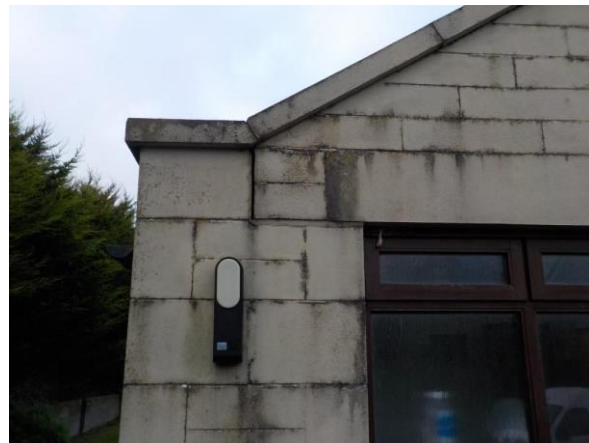
Open joints southeast side.
