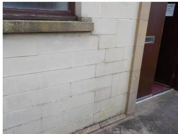
Joint cracking east gable.
