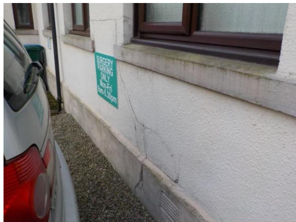
Cracking to west end.
