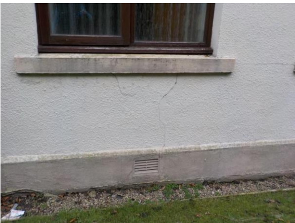
Cracking to south elevation.
