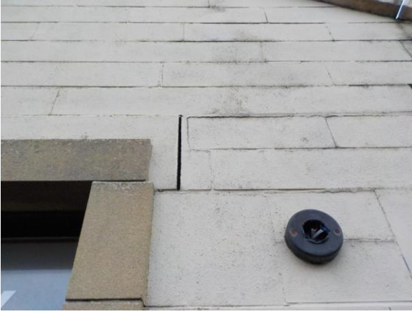
Open joints northeast side.
