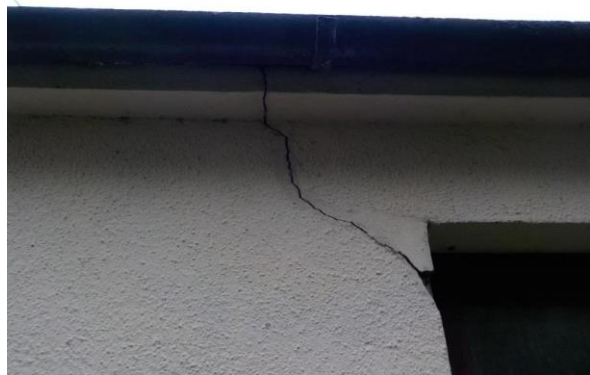
Cracking to west end.
