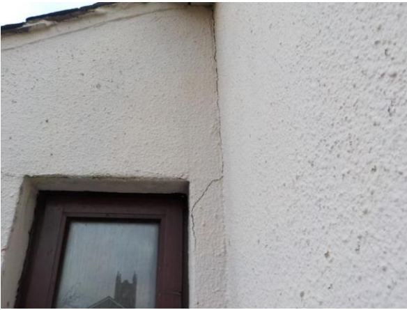
Cracking of side extension east end.
