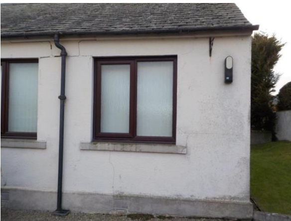
Cracking to west end.
