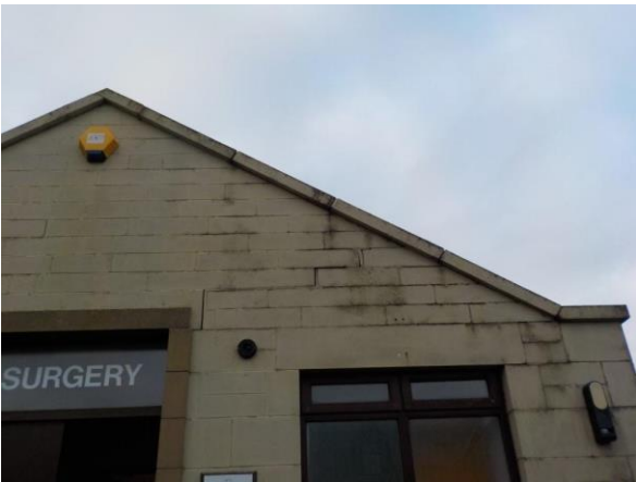
Open joints northeast side.
