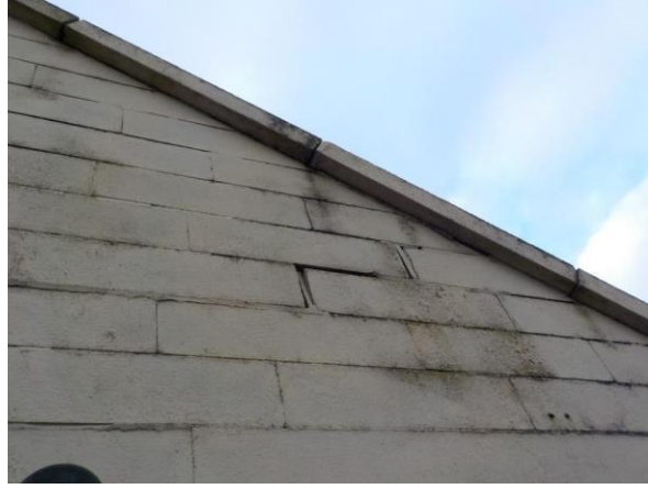
Open joints northeast side.
