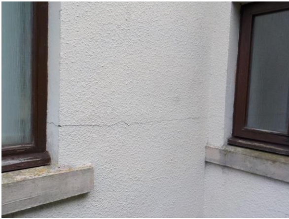
Cracking to east end.
