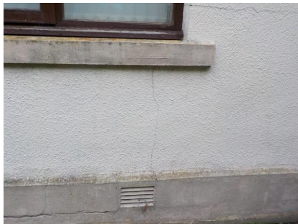
Cracking to south elevation.
