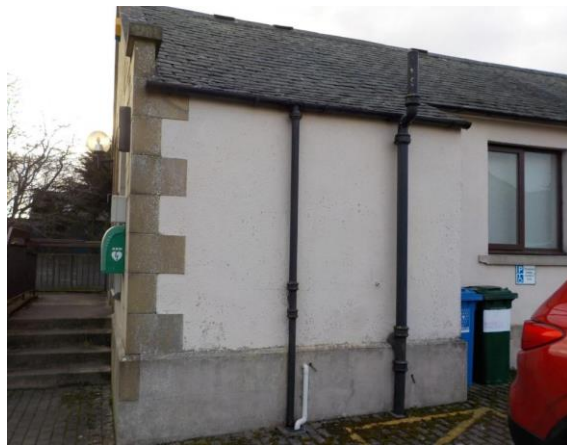
External view of sagging roof.
