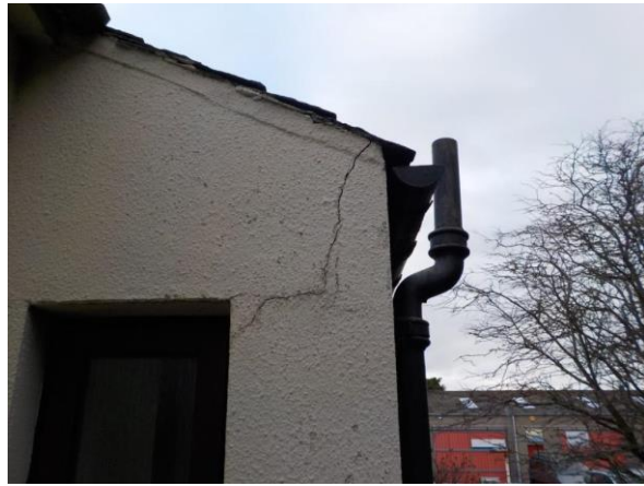
Cracking of side extension east end.
