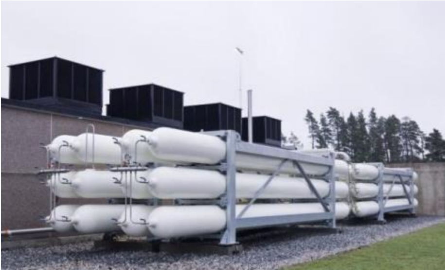
Figure 9.3: Hydrogen Tube Rack High Pressure Storage
