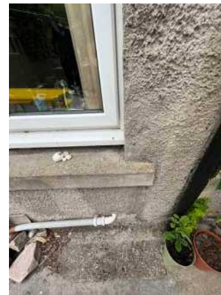
019 south elevation kitchen window concrete sill
