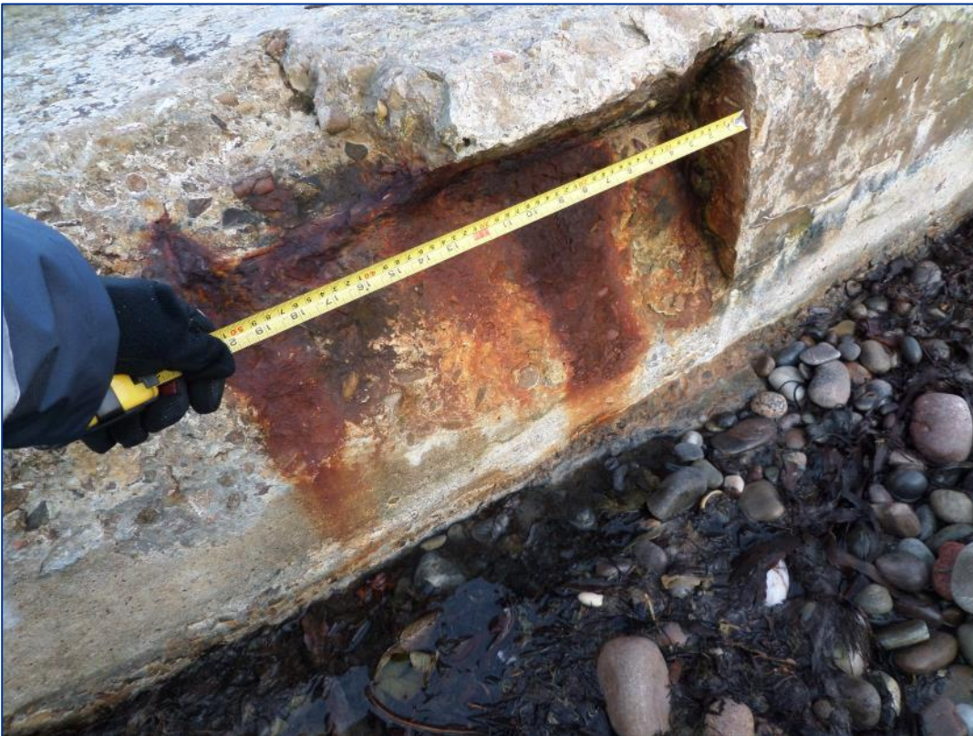
Figure 2-6: Rust-staining to concrete wall (2016).
