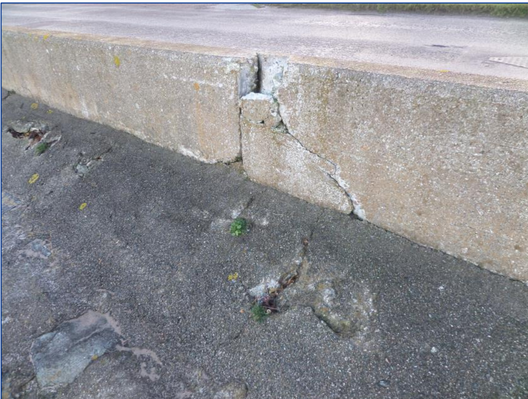
Figure 2-12: Further damage and cracking to setback wall (2016).
