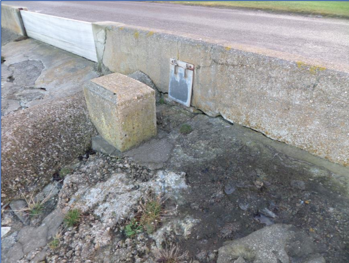
Figure 2-13: Flap valve and gap in the wall blocked off by wooden planks (2016).
