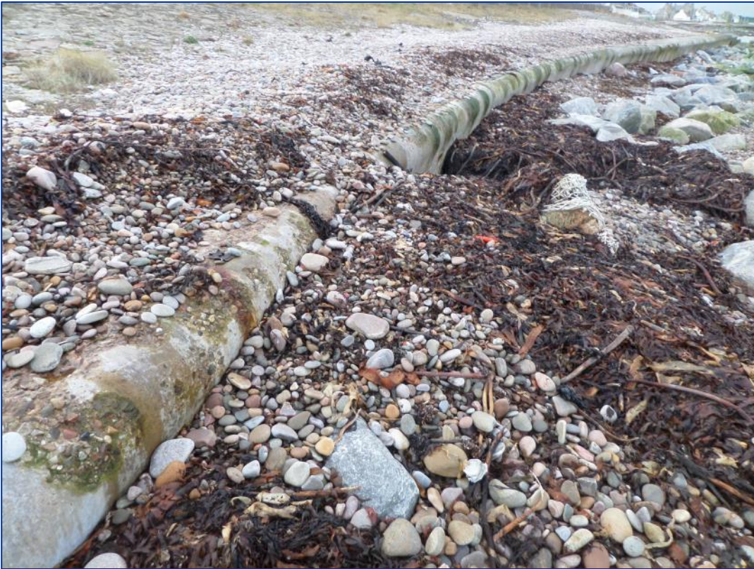
Figure 2-4: Rock armour has slumped and is partially buried at the western end of the coastal defences (2016).
