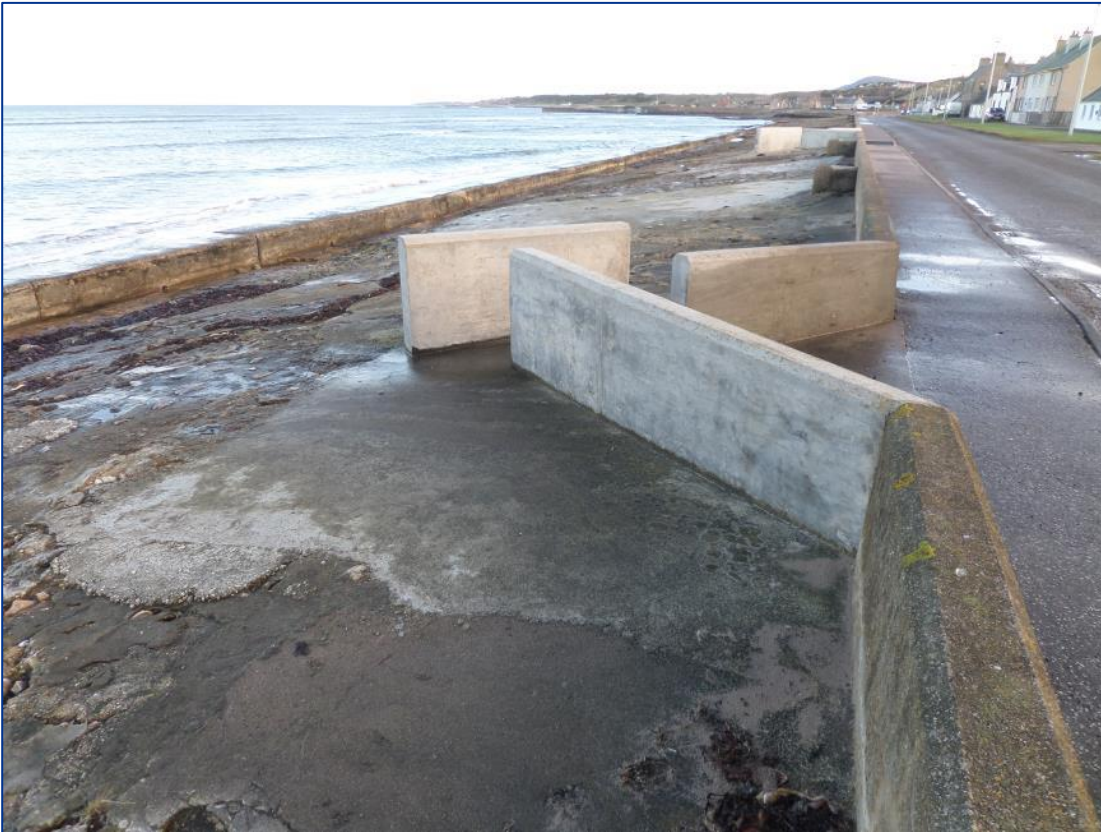
Figure 2-14: View looking towards the Harbour end of the coastal defences, showing the older baffle arrangement in the foreground and the newer arrangement further along the setback wall (2016).
