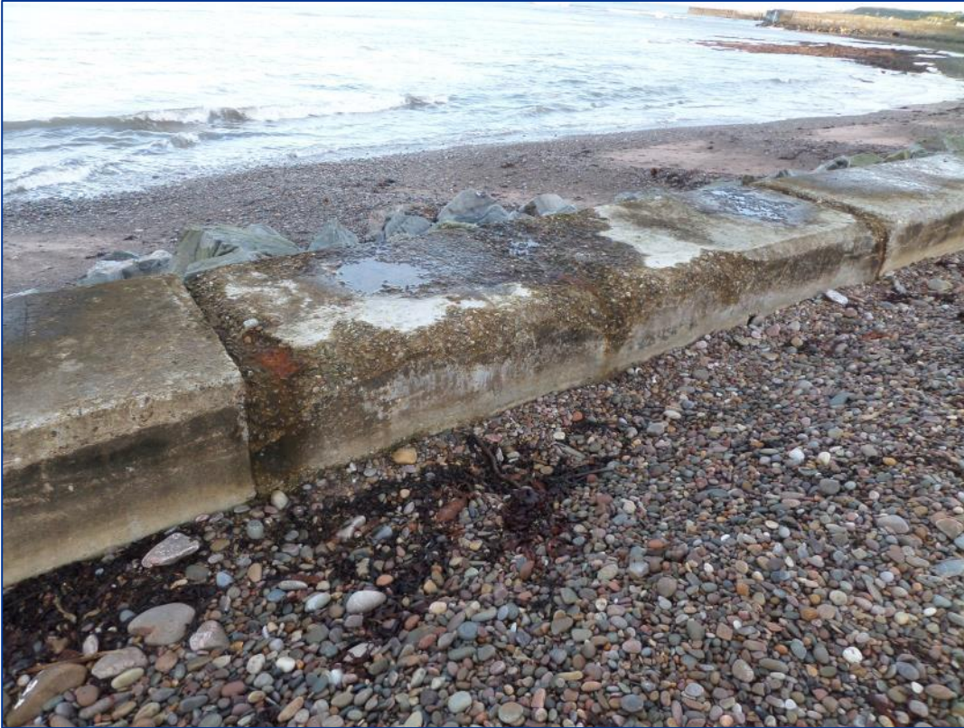
Figure 2-5: Spalling of concrete wall, exposing aggregate (2016).
