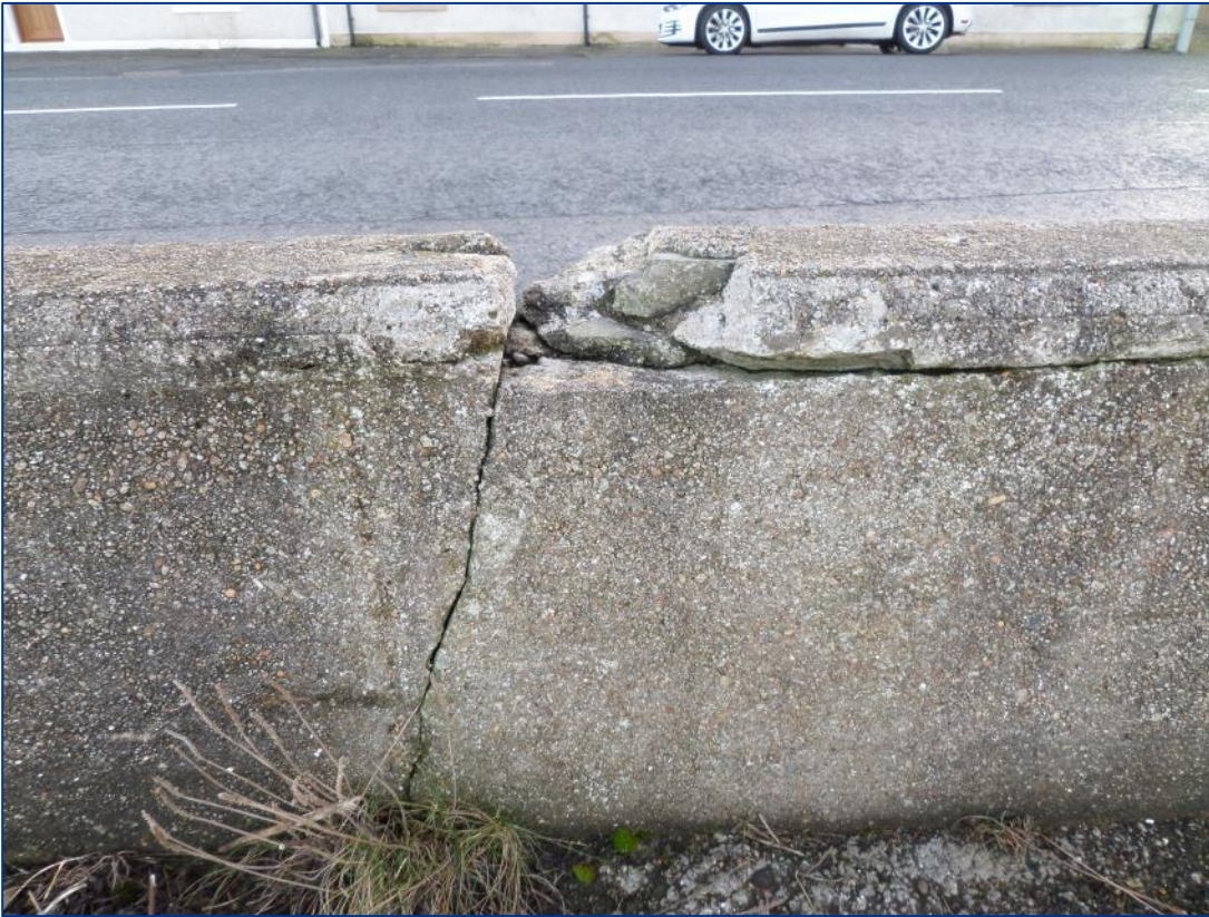
Figure 2-11: Damage to crest and cracking of the setback wall (2016).
