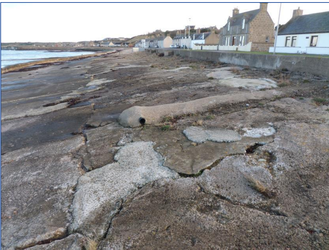
Figure 2-9: Extensive concrete patch repairs. Drains are placed periodically along the length of the wall (2016).
