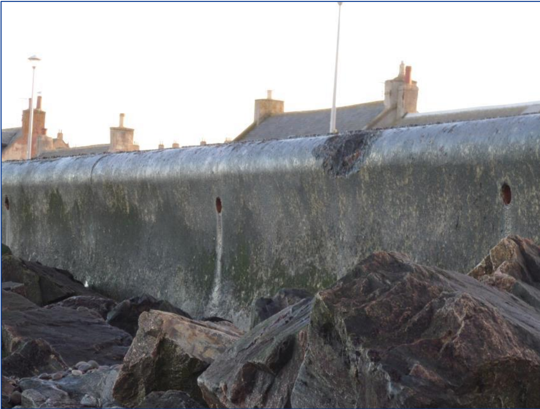
Figure 2-7: Damage to face of wave return wall (2016).
