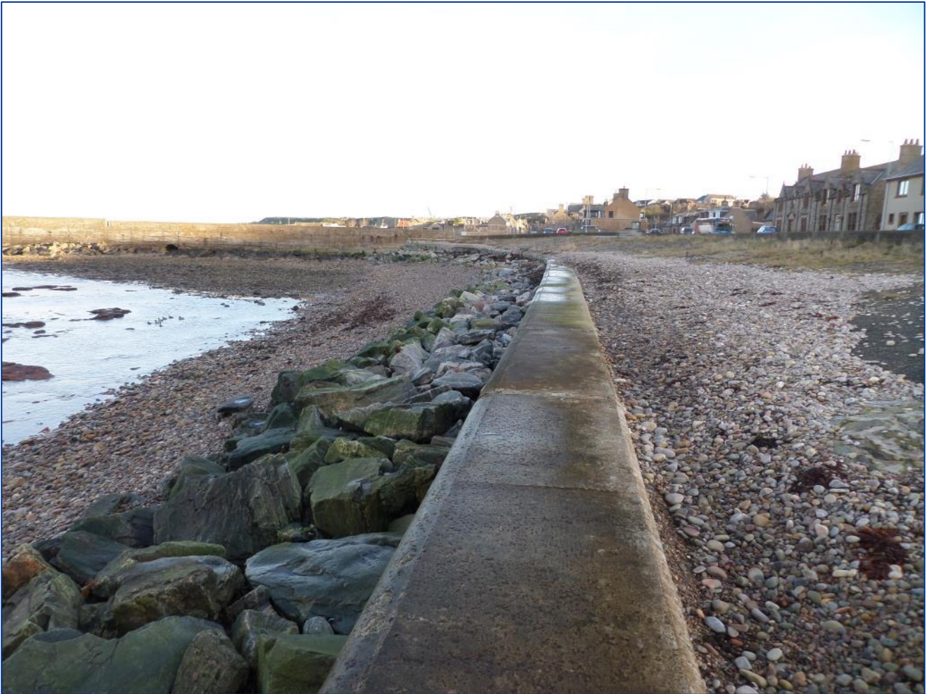
Figure 2-3: View of rock armour at the east end of the defences, showing significant burial of the rock slope to the left of the wall and significant deposition of pebbles on the right of the wall (2016).
